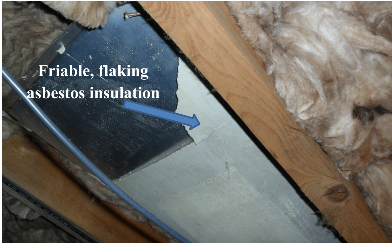
Figure 4-3: Asbestos Duct Insulation in Basement Ceiling
