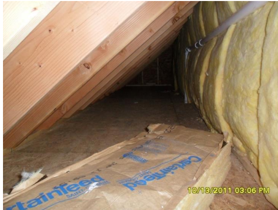
Figure 28: Grade III Fiberglass Batts—Attic Kneewalls in Newly Constructed Home
