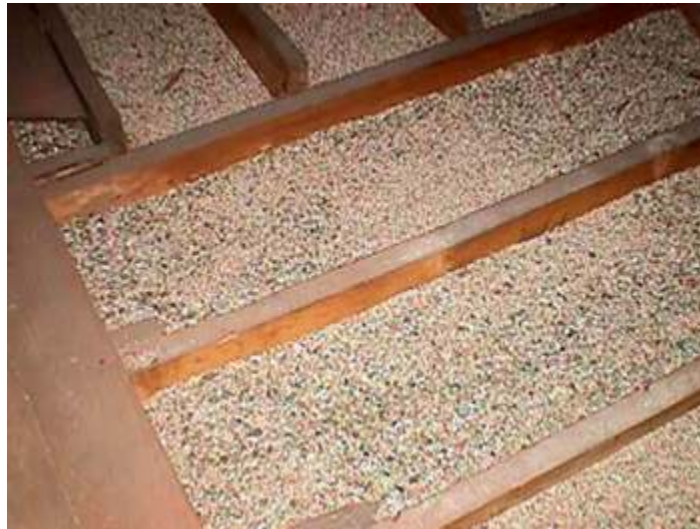
Figure 4-4: Vermiculite Insulation between Attic Rafters
