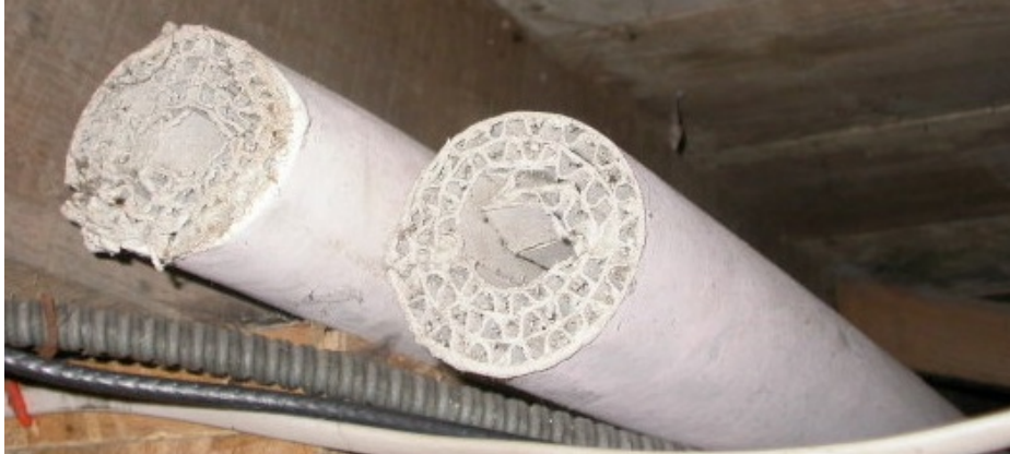
Figure 4-1: Asbestos Pipe Insulation - Dangerous
