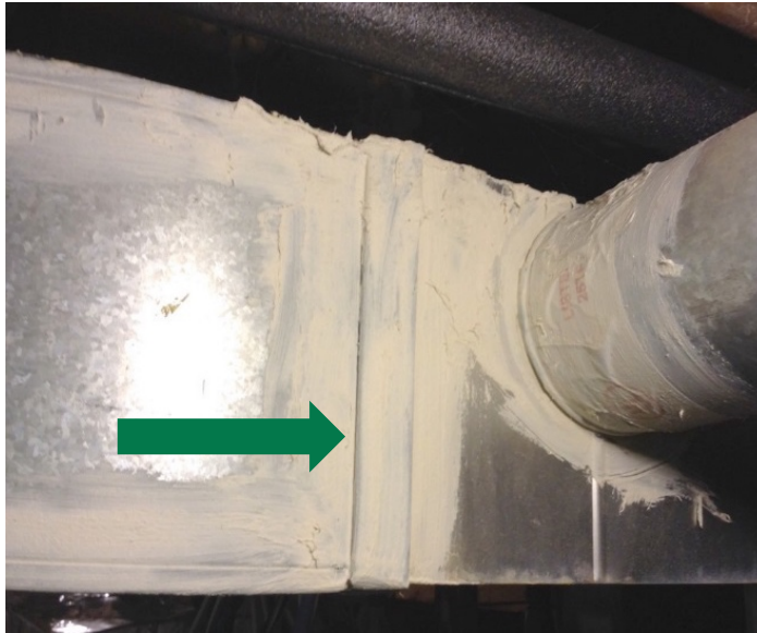
Figure 17: High-Quality Duct Sealing with Mastic
