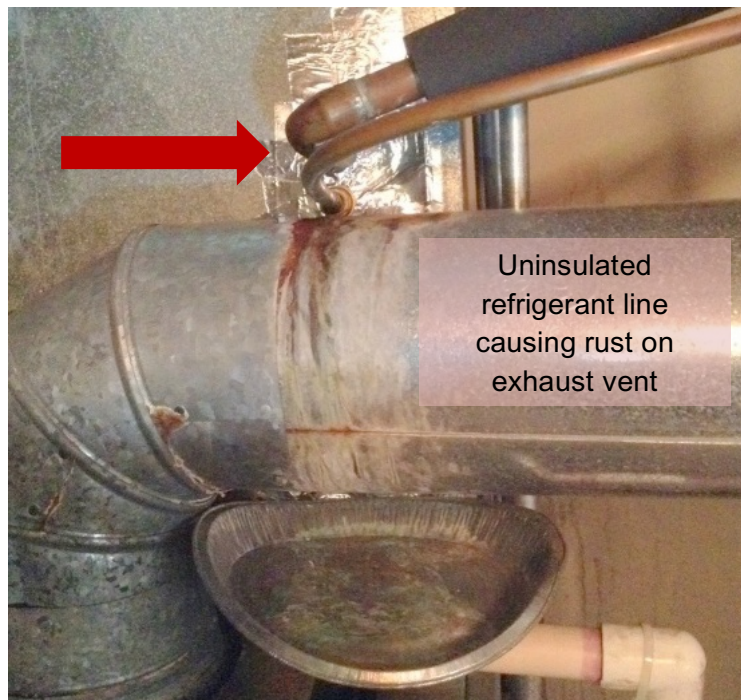
Figure 19: Future Health and Safety Issue – Condensation Rusting Exhaust Vent
