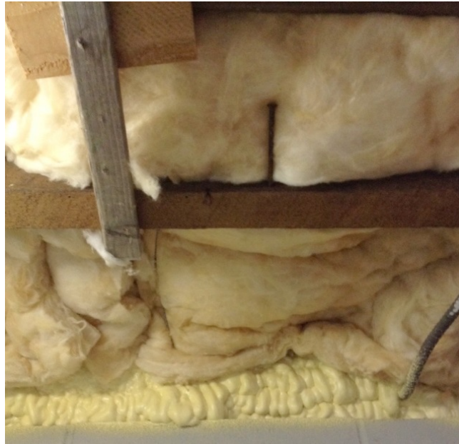
Figure 7: High Quality Rim Joist Air Sealing and Low Quality Basement Ceiling Insulation
