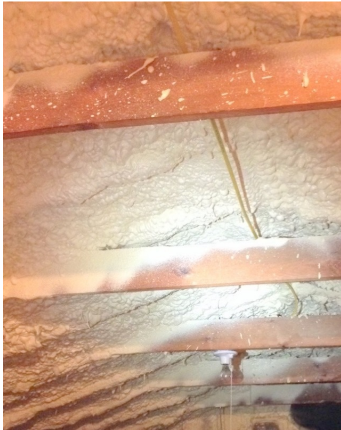
Figure 8: High Quality Attic Insulation with Spray Foam
