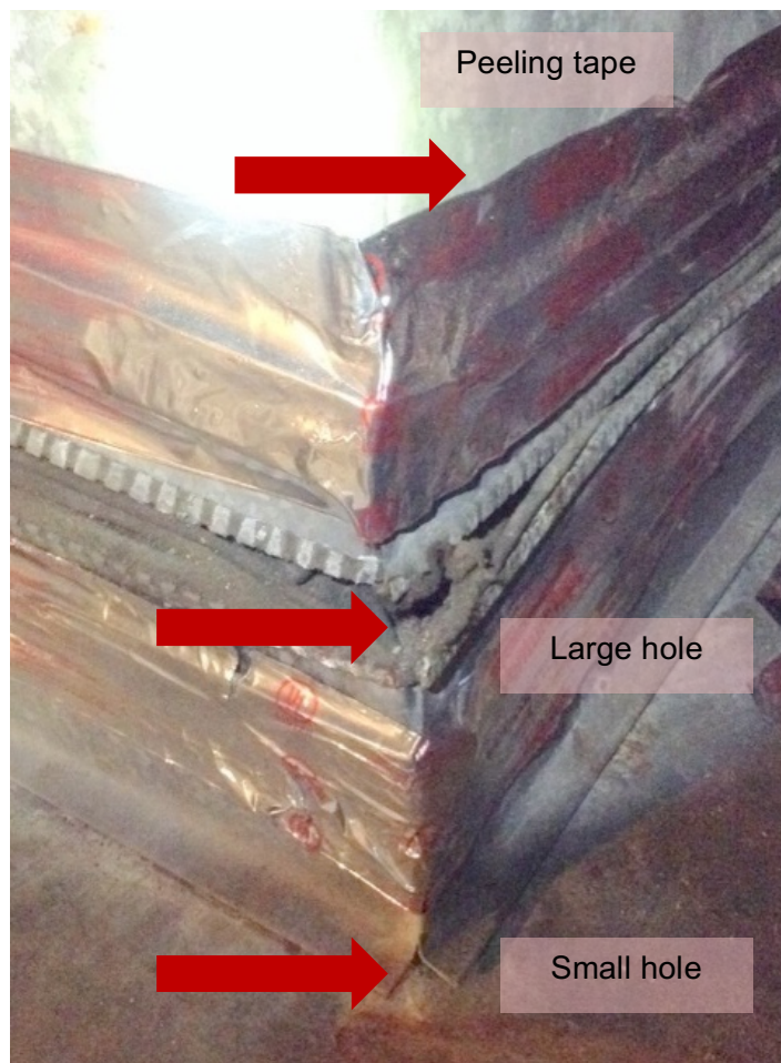
Figure 15: Poorly Sealed Ducts
