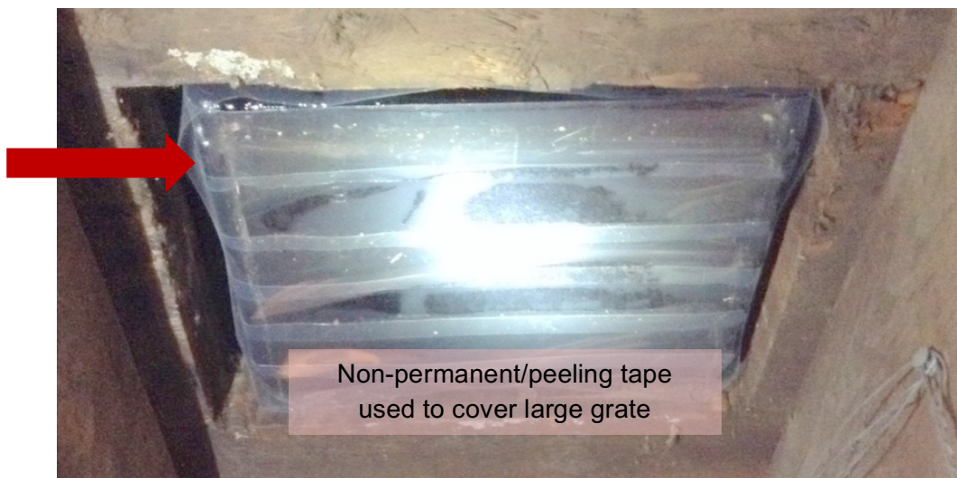
Figure 14: Inappropriate Basement Ceiling Air Sealing
