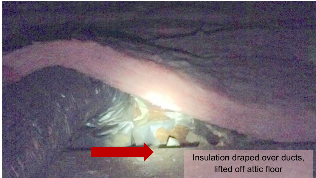
Figure 24: Low-Quality, Non-HES Attic Insulation
