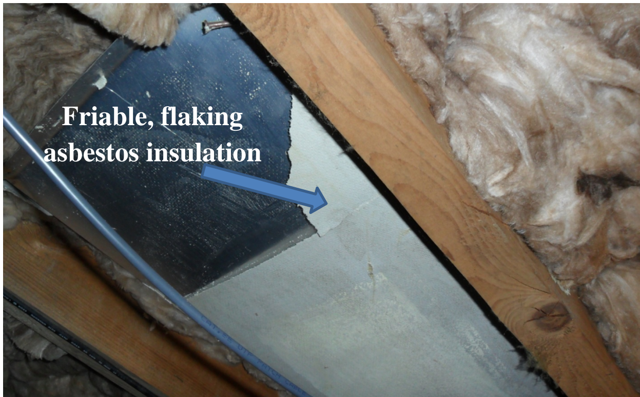
Figure 4-3: Asbestos Duct Insulation in Basement Ceiling
